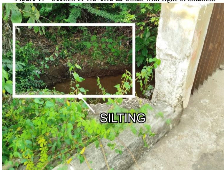
Figure 11 - Section of Travessa da União with signs of siltation.
